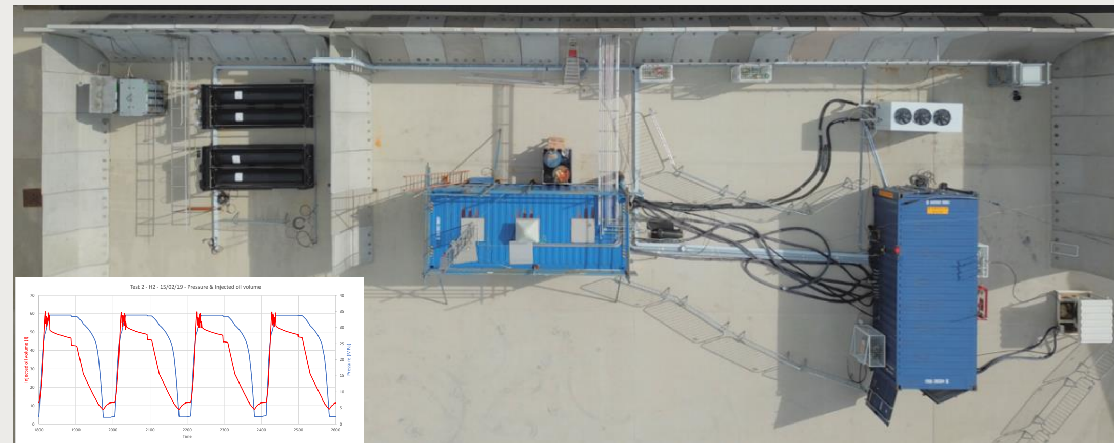
Aerial view of hydrogen test area for full scale CBM testing in closed loop
